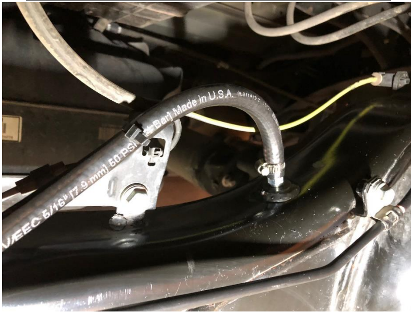
Figure 2 – Jomax Customs Relocation Installed at Differential Note - Surface area cleaned before installation
